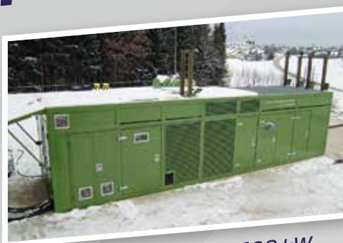
Mobiles Dieselaggregat 1600 kW
